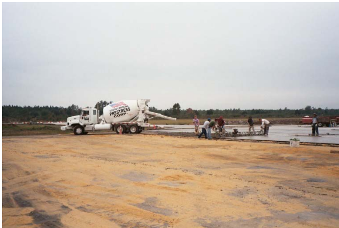
Photo 3: Sand use as a crack filler and to act as a bond breaker for Williamsburg County Regional Airport whitetopping.
