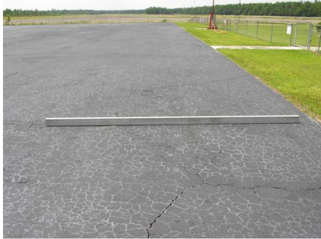
Photo 2: Condition of Williamsburg County Regional Airport Apron before whitetopping
