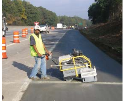
Within the first two hours of placement, an early entry (Soff-Cut) saw cuts contraction joints to match the adjacent mainline pavement.
