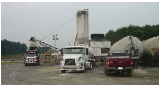
The RCC material is being manufactured on-site in a continuous pug-mill operation. This unit, an Aran ASR280B, produces RCC at rates of up to 500 tons per hour.
