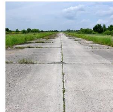
Joint Sealant Failure
