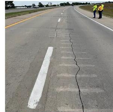
Low-Severity Longitudinal Cracks or Joints
