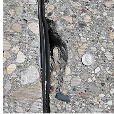
Spalled Joints and Cracks
